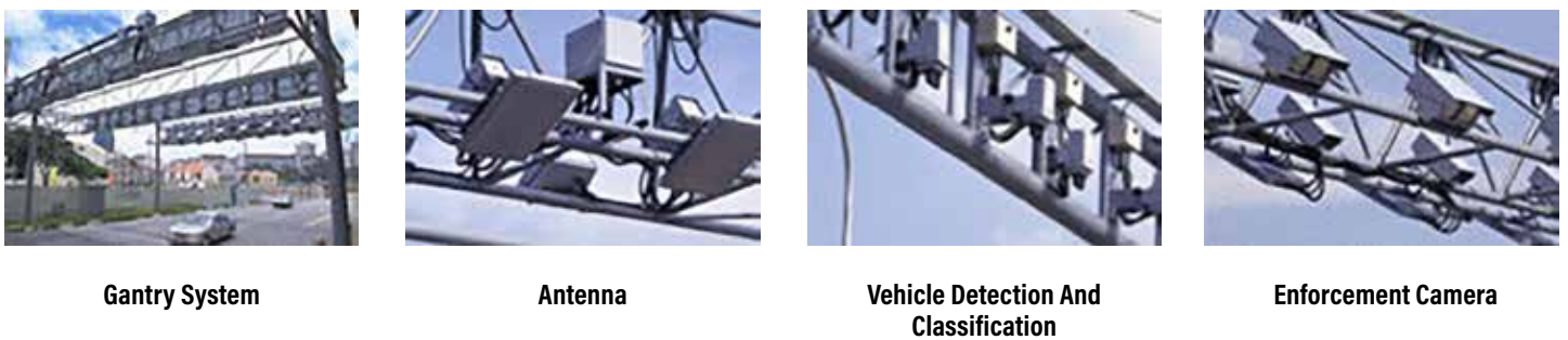
Figure 4-10 | Charging System on ERP Gantry
